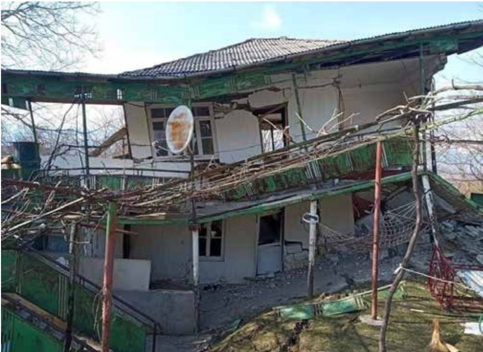
Destroyed House in Itkhvisi, Chiatura. (Photo: Radio Liberty)
