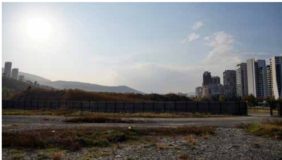
Construction of a new park on the site of the former hippodrome in Tbilisi. (Photo: Radio Liberty)
